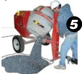
5 Mix for 6 additional minutes (7 minutes total) and place. Pour DOTline™ into repair site. DO NOT RE-TEMPER WITH WATER
