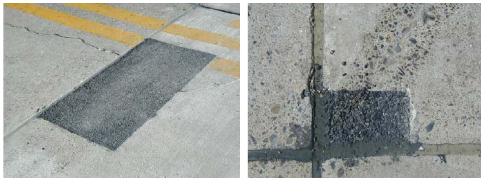
Figure 3: Failure of cold asphalt repairs; settlement due to heavy traffic loads and tearing of patch due to torsion
