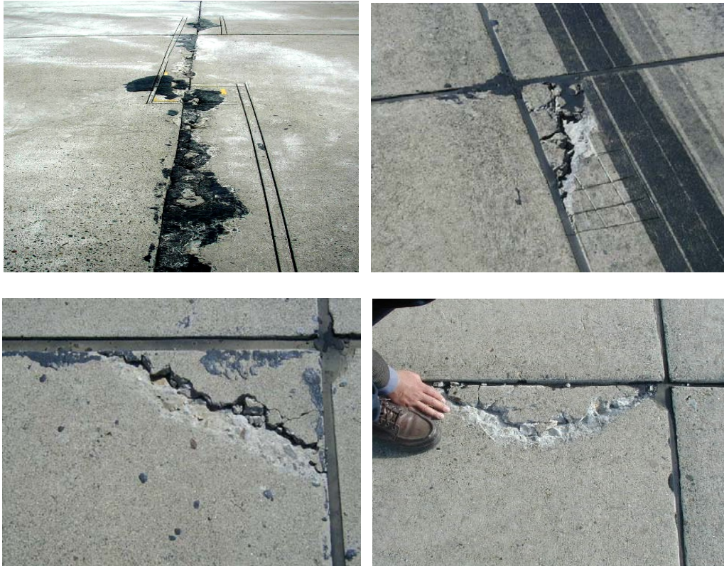
Figure 1: Examples of Condition 2 in slabs of PCC pavement
