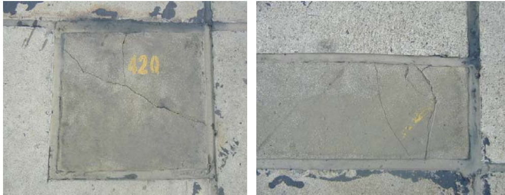
Figure 6: Cracking of patches completed with epoxy compounds
