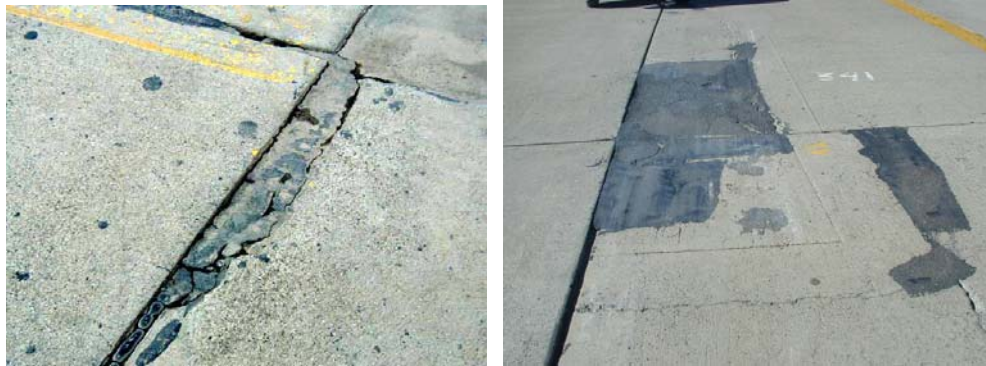
Figure 2: Failure of hot asphalt repairs on PCC pavement
