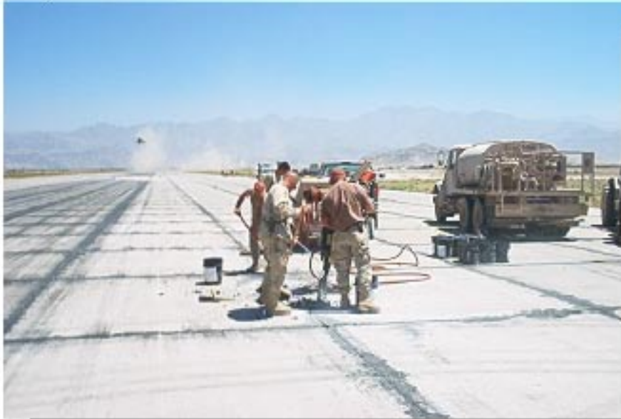
Figure 10. AFRL / MLQD personnel instruct an Air Force RED HORSE team on the use of PaveMend TM , a chemically-bonded fly ash repair material, at an undisclosed location during Operation Enduring Freedom.
